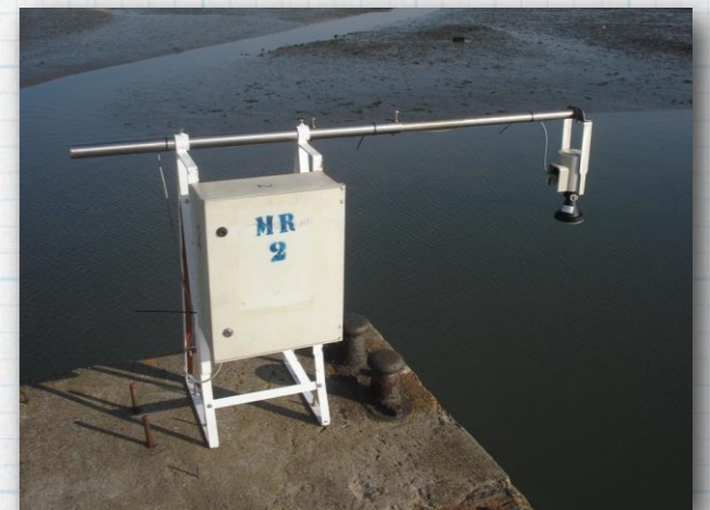
Radar Tide gauge.
